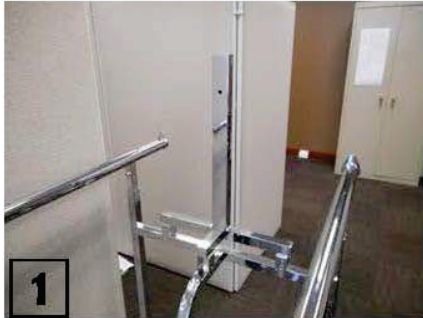
Saddle "Upright Bracket" over the existing H-Rack
