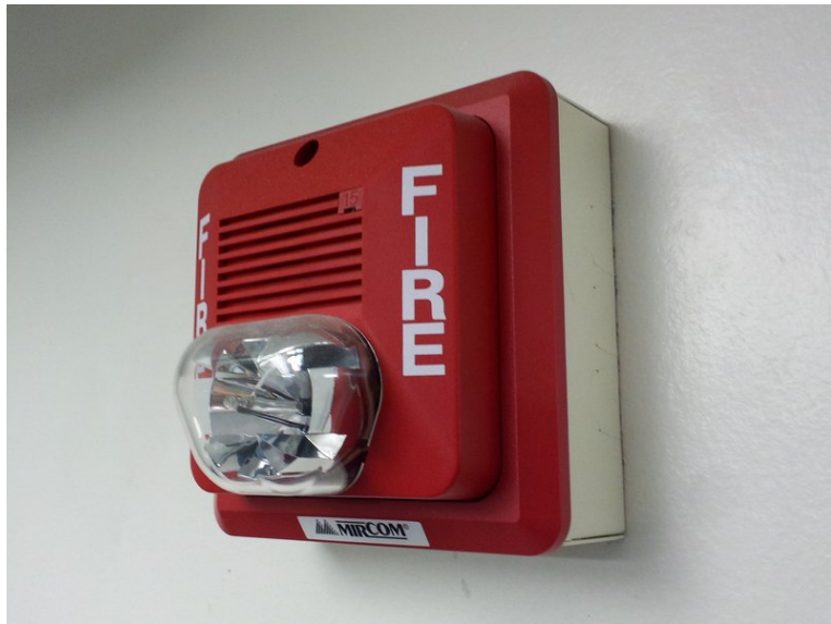
Strobe smoke alarm
