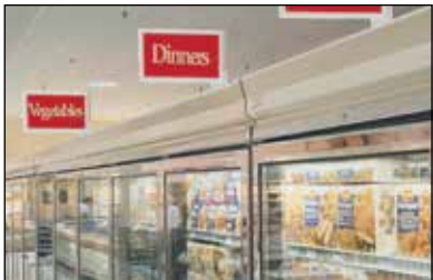
RAZZ® on top of coolers
