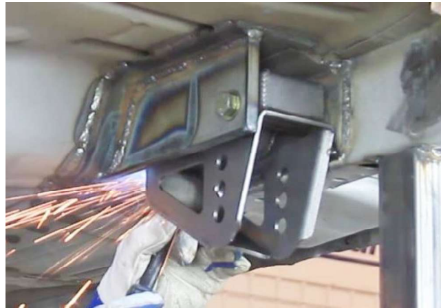
Figure 17 - Weld Front Lower Link Bracket
