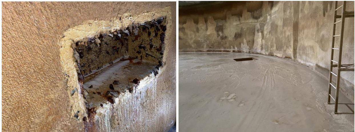
Figure 13: Examples of lime sludge found inside a ground storage tank. On the left is sludge buildup at a side access port. On the right is a tank floor with a couple of inches of sludge.
