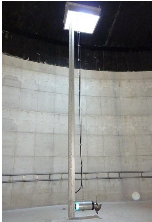
Figure 10: A rail-mounted submersible mixer which is removable from the hatch above.
