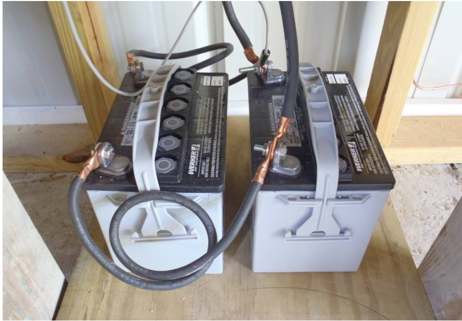
A dry easily accessible location for the batteries
