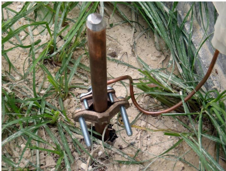
Grounding rod with the grounding wire securely fastened
