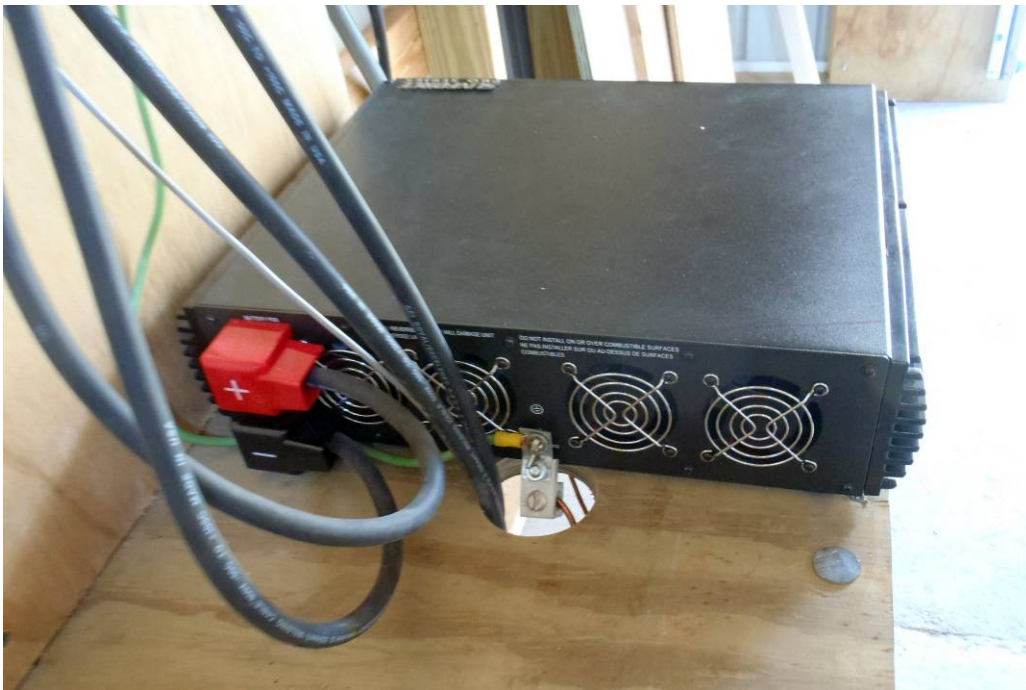
DC Connections in the rear of the SunForce Inverter
