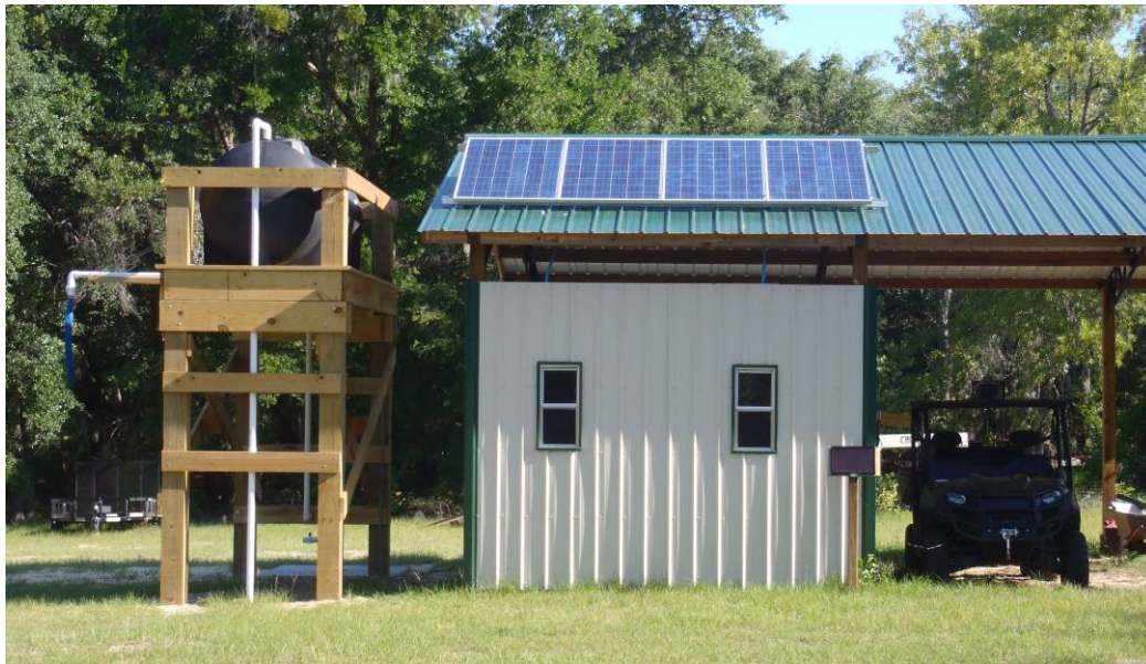
The finished installation of the solar panels
