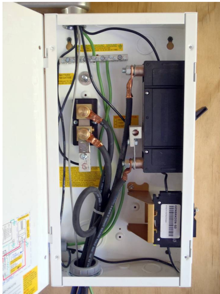
Electrical Disconnect Box wiring
