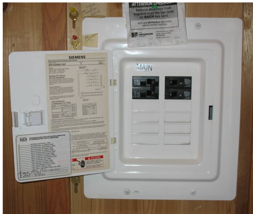
Circuit Breaker Box
