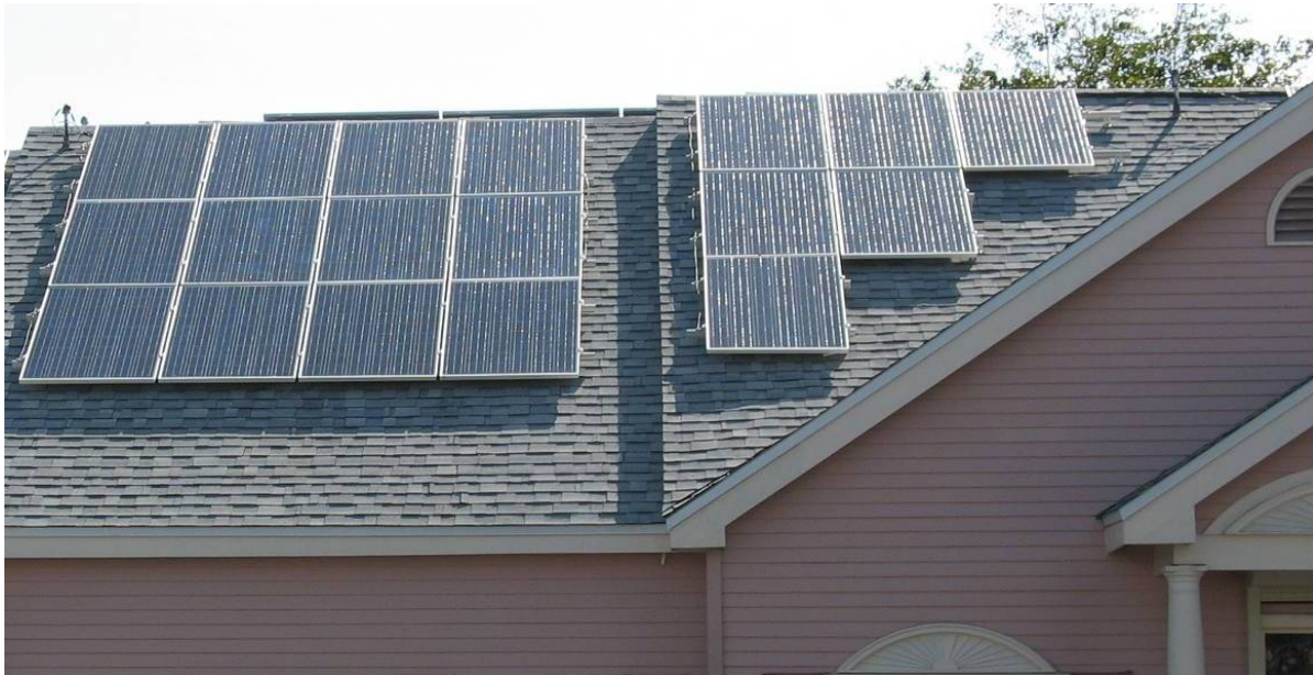
Figure 10 – Roof-mounted solar panels
