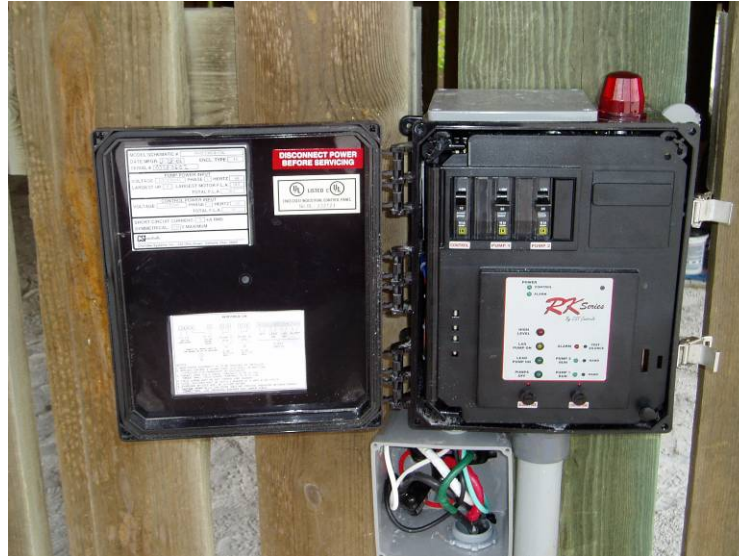
A control panel
