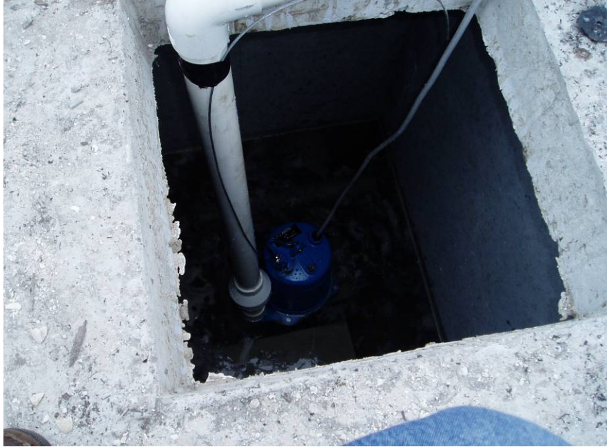
A septic dosing pump installed in a tank
