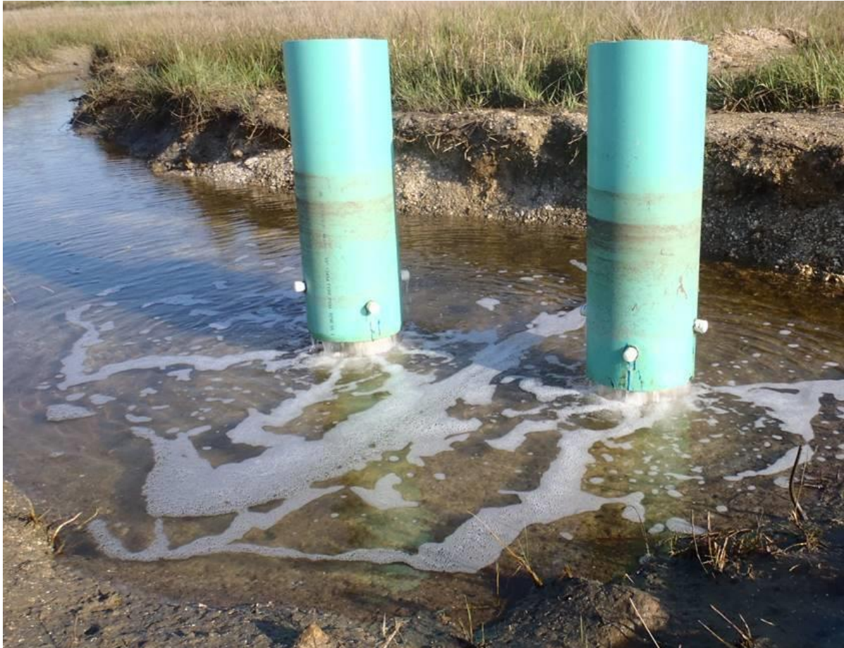
Figure 10 – Two of the 4 Bi-directional Flow Pipes shown when discharging from the Pond into the Marsh. The brown stains indicate the various high tide elevations.
