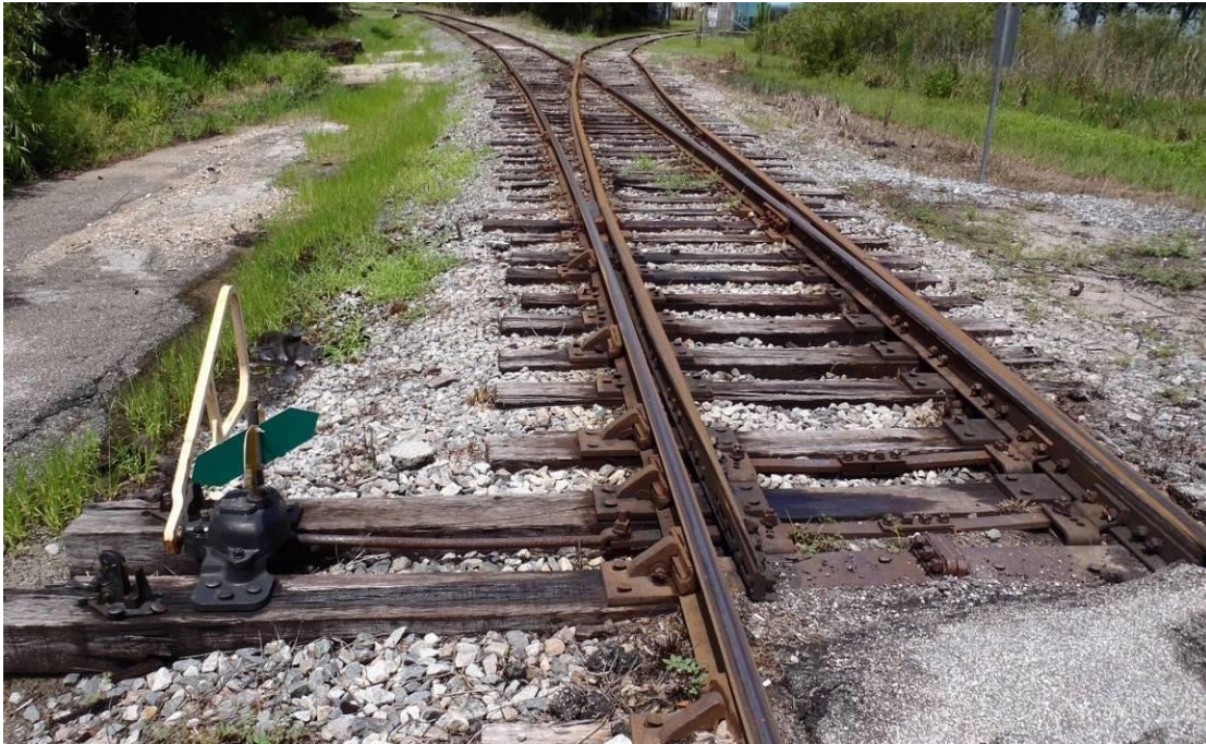
Figure 22 – A manual switch with a turnout for a customer's facility
