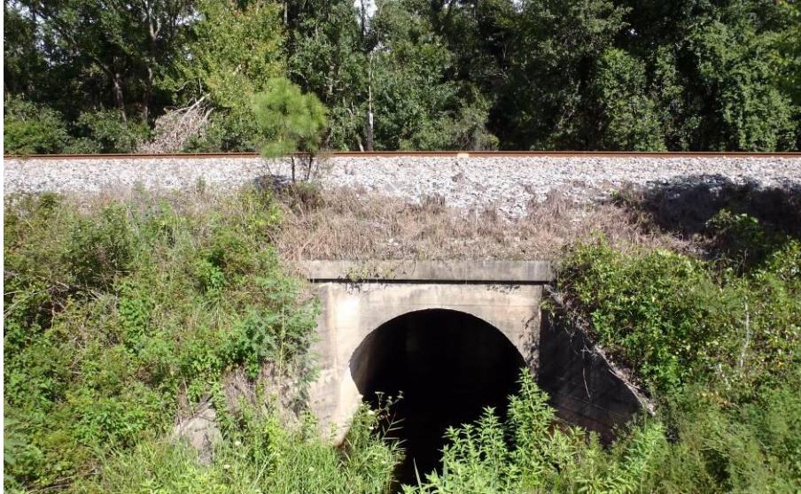
Figure 13 – Rail drainage system using a round culvert
