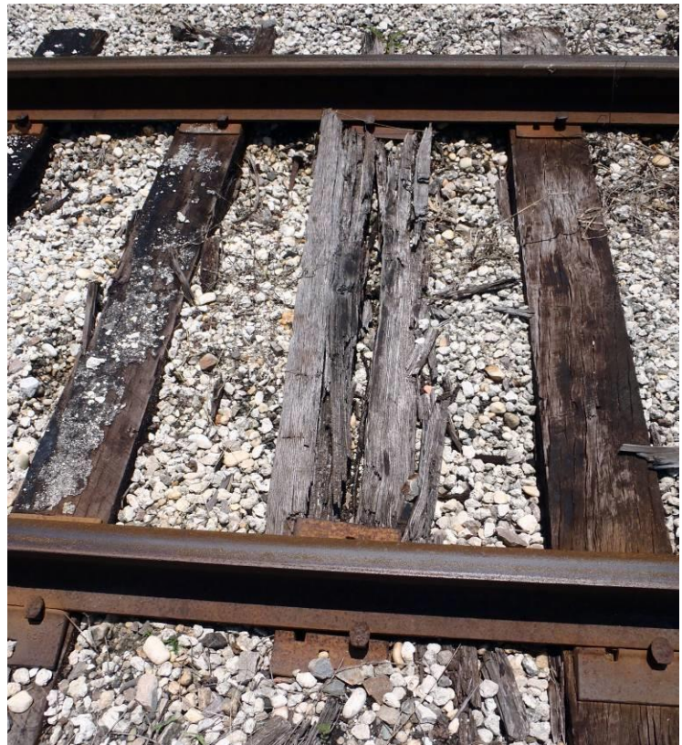
Figure 16 - Railroad Ties – The good and the bad
