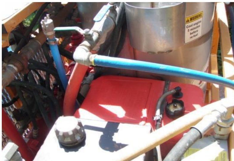
Figure 23 Water enters the mixing hopper as controlled by the valve.
