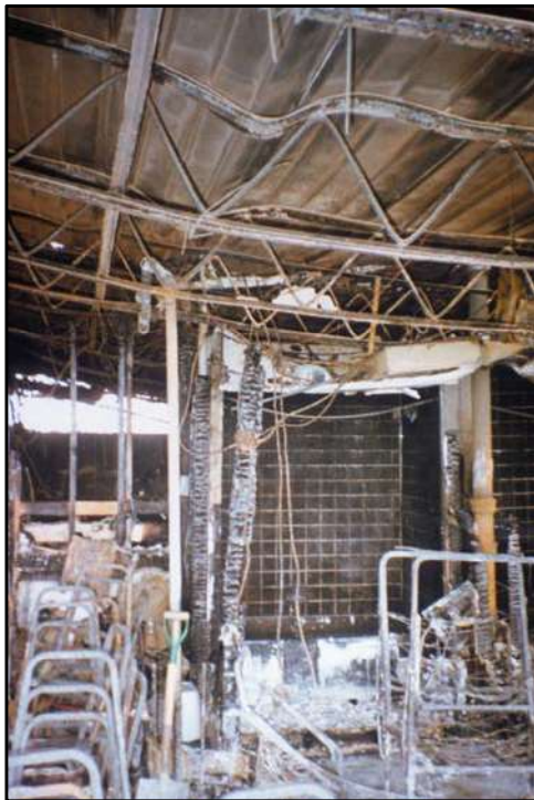
Photo No. 11 - Steel bar joists after a fire. Notice buckled top chord.
