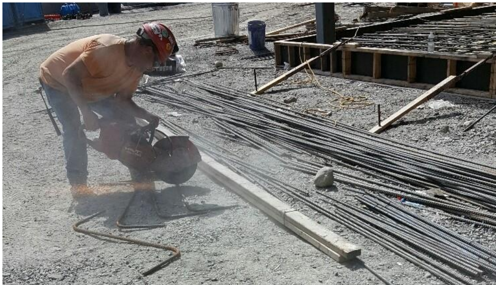
Field cutting rebar with corresponding sparks and danger nearby
