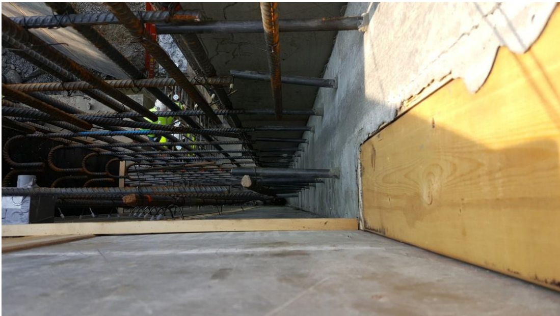
Rebar was too short against smooth dowels without overlap.
