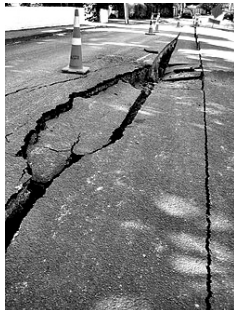
Earthquake Damage - Roads Christchurch, NZ
