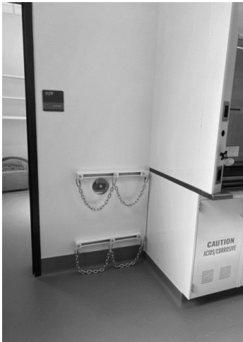
Gas cylinder tank supports on a wall adjacent to a fume hood
