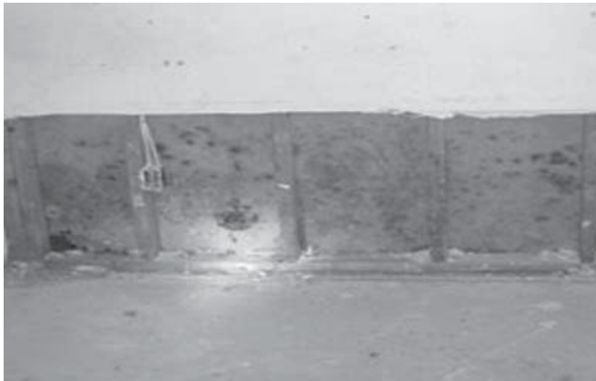
Mold on the back side of drywall
