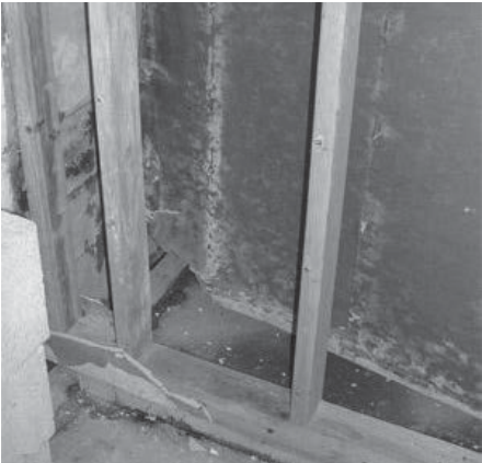
Mold inside a wall cavity
