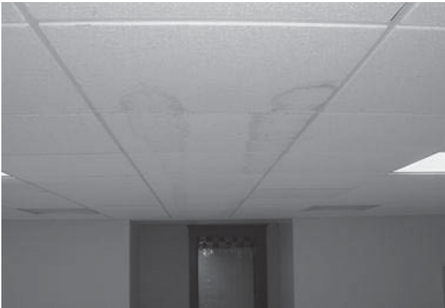
Water stained ceiling tile
