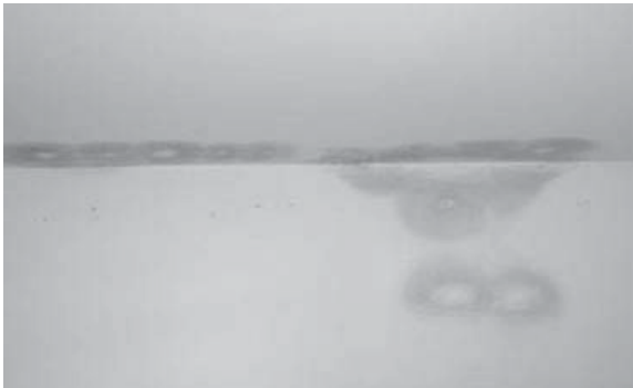
Water stains on drywall
