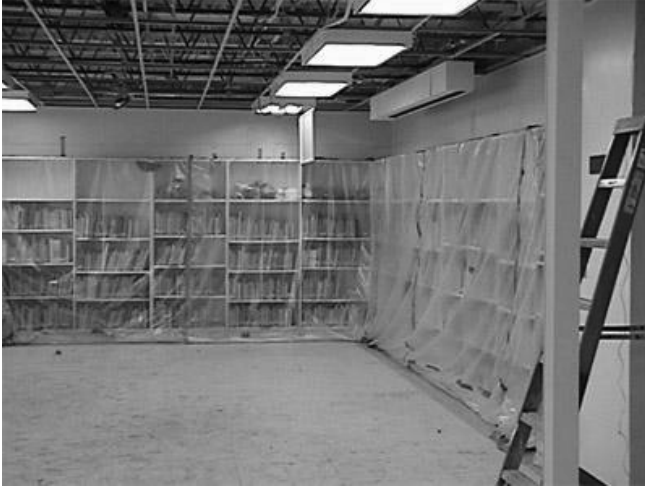
Minimizing further damage during restoration
