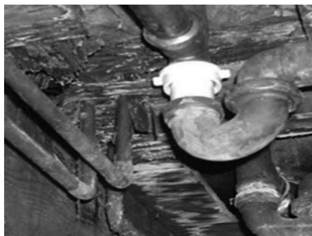
Mold growth because of bathtub leak
