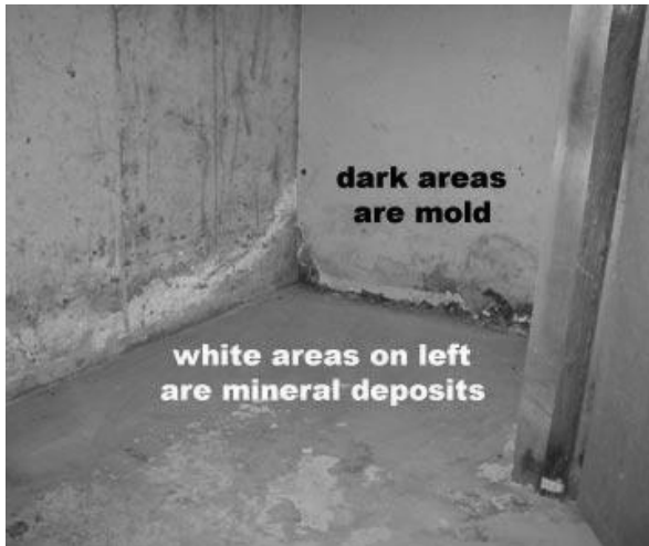
Water penetrating through foundation walls
