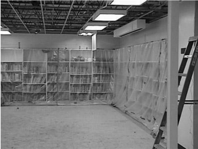
Minimizing further damage during restoration
