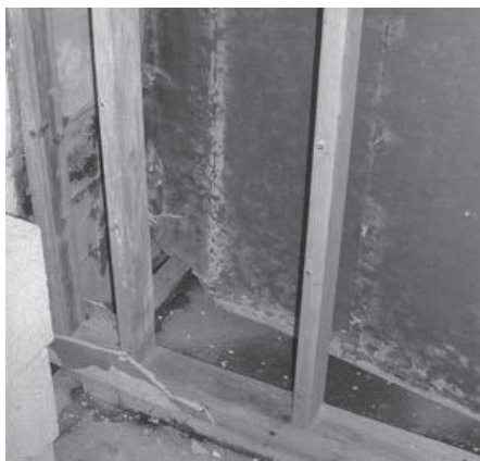
Mold inside a wall cavity
