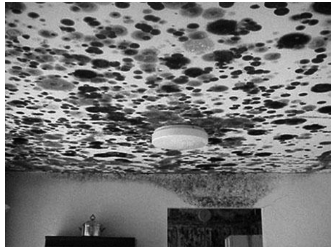
No testing to verify mold, needed here
