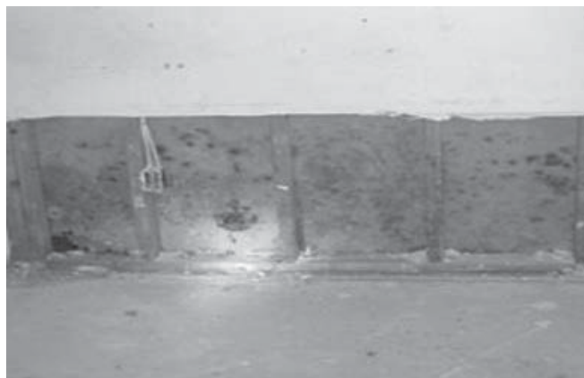
Mold on the back side of drywall
