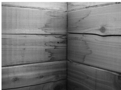
Permanent water stains on wood
