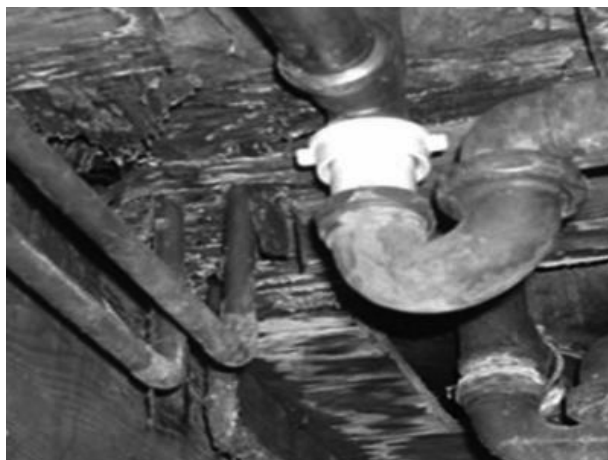
Mold growth because of bathtub leak
