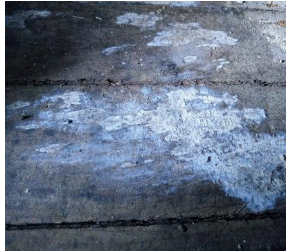
Mold Heralding a Moisture Problem
