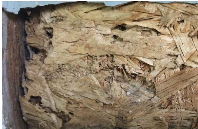
Damage from Water Absorption
