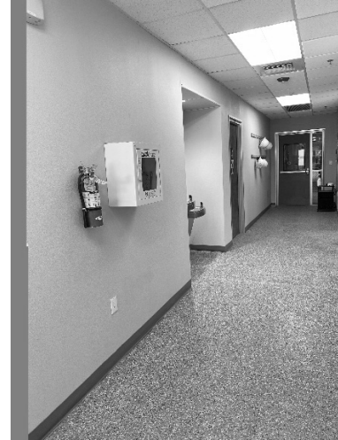
Protruding Objects – AED Cabinet and Fire Extinguisher
