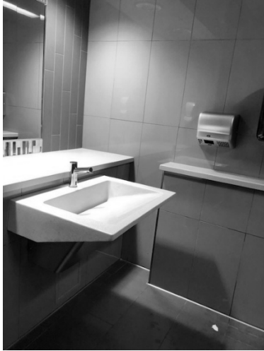
Protruding Object – Sink
