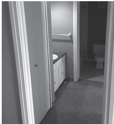
Seriously Inaccessible Bathroom
