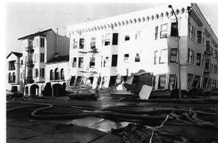
Earthquake damage in San Francisco's Marina District on the north side of the city from the Loma Prieta Earthquake October 17, 1989.
