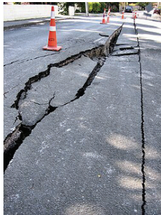
Earthquake Damage - Roads Christchurch, NZ
