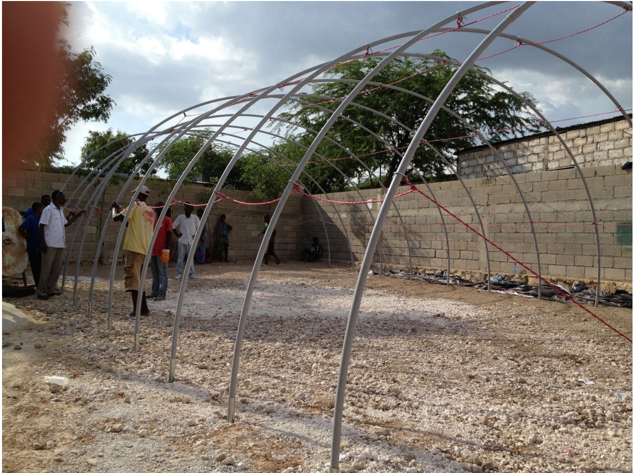
The ribs of the frame were held in position with ropes that maintained the spacing and stabilized by guying to posts driven into the ground.
